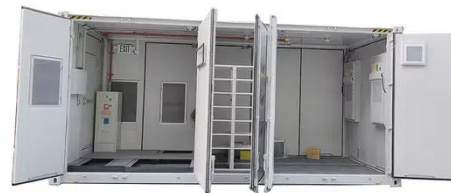
1075KW HH ESS
